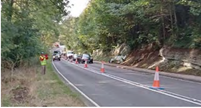
The Warwickshire County Highways traffic control system in action on Blackford Hill on the A4189 near Henley-in-Arden. The cars parked on the right, behind the cones, belong to the WGCG workforce clearing the Arden Sandstone exposure. Photo by Max Down, WGCG
